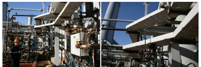
Figure 7: Photos of the GINSENG deployment.
