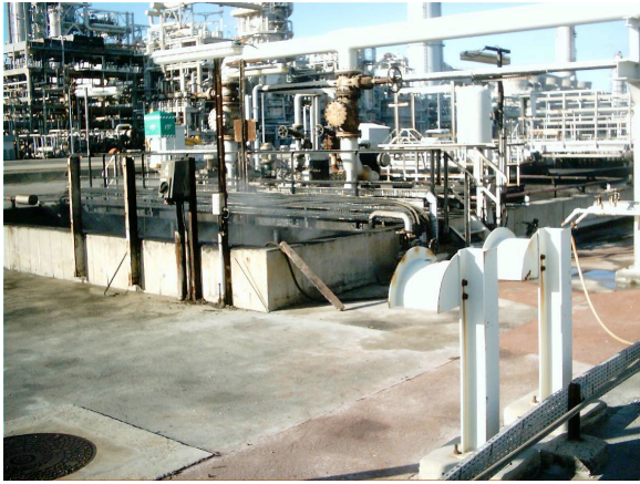
Figure 2: Water treatment area - Line 4.
