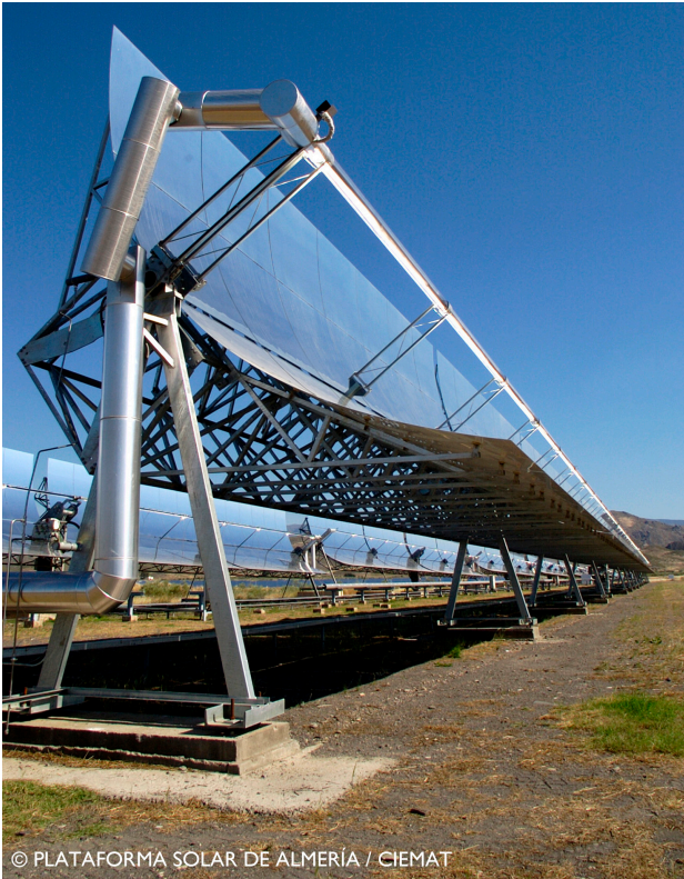
Fig. 3. Acurex solar collector loop.
