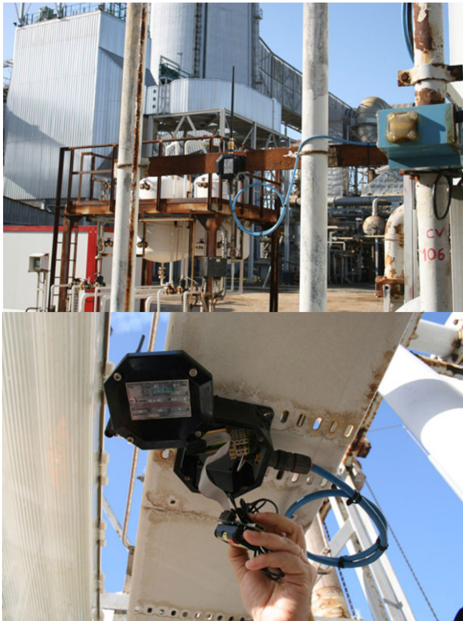
Fig. 10: Sensors deployed in the refinery.
